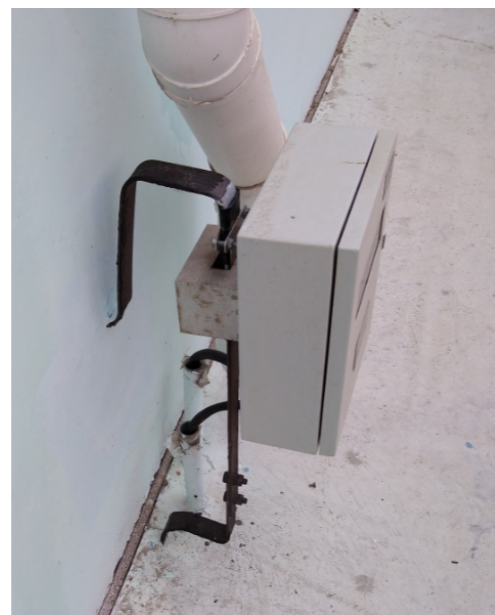
Explosion-proof grounding resistance detector site
